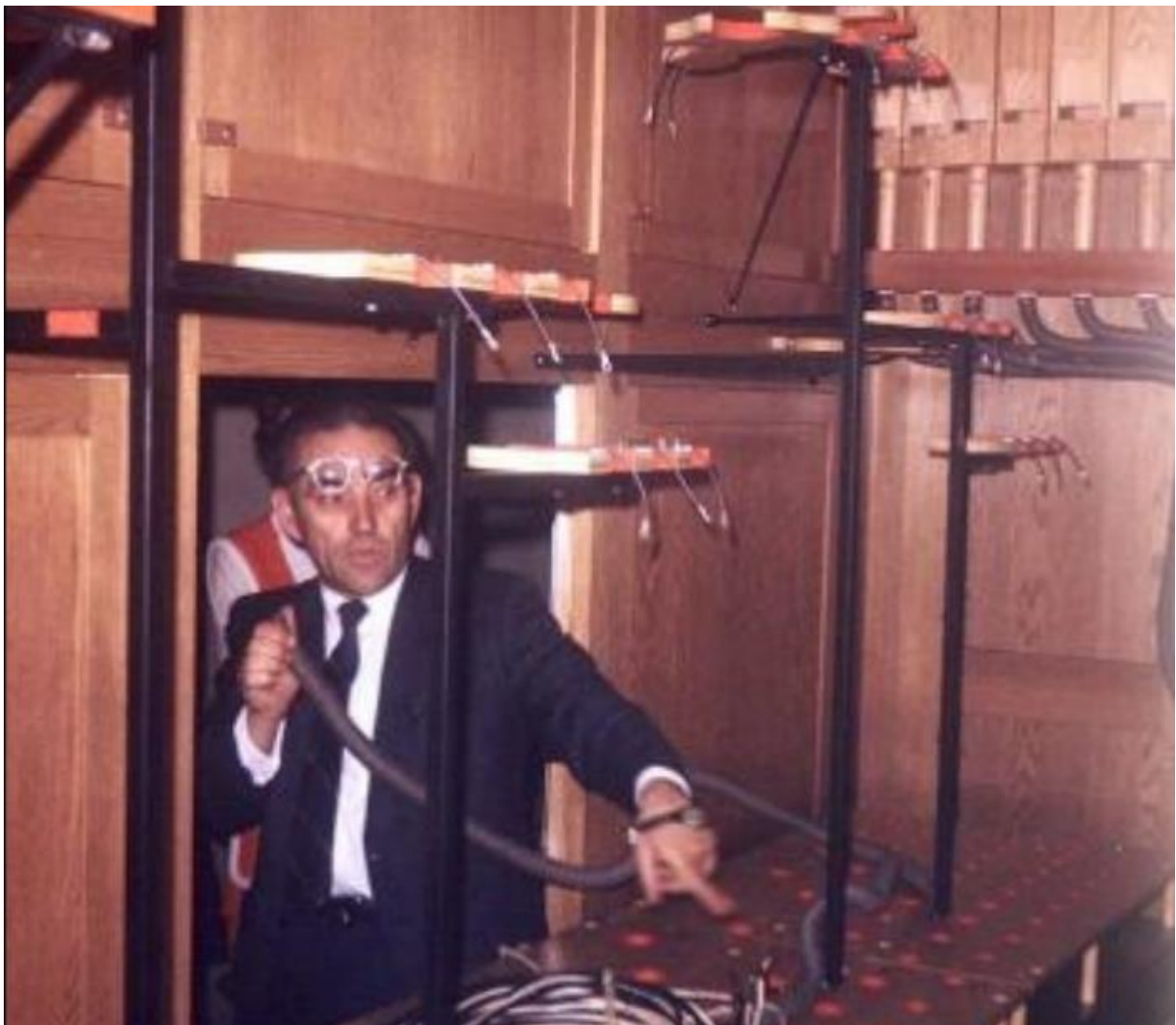
Krapf inspecting the organ installation at the University of Iowa's Clapp Recital Hall. (Jeff Charis-Carlson, "Remembering Gerhard Krapf: A History Behind St. Andrew's 'New' Organ," The Messenger of First Presbyterian Church [Iowa City, Iowa], October 2018.) 4-5.
